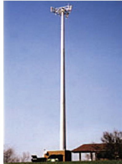
Figure 10: The application of the 100% solids rigid aliphatic polyurethane on a galvanized steel communication tower.
