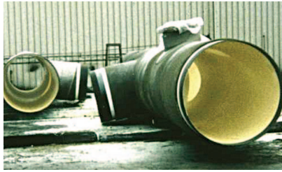
Figure 8: The application of a highly abrasion resistant 100% solids rigid polyurethane lining on a 36" steel pipe for extremely high water flow rate.
