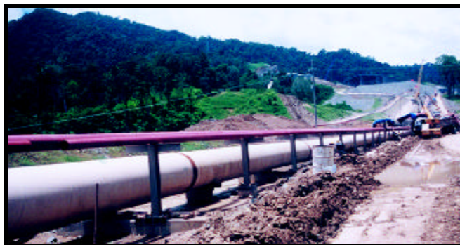
Over five miles of 54 inch diameter above ground seawater steel pipeline, lined and coated with Madison's polyurethane.
