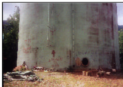
Double Gate 500,000 Gallon Ground Storage Water Tank Seriously in Need of Rehabilitation!
