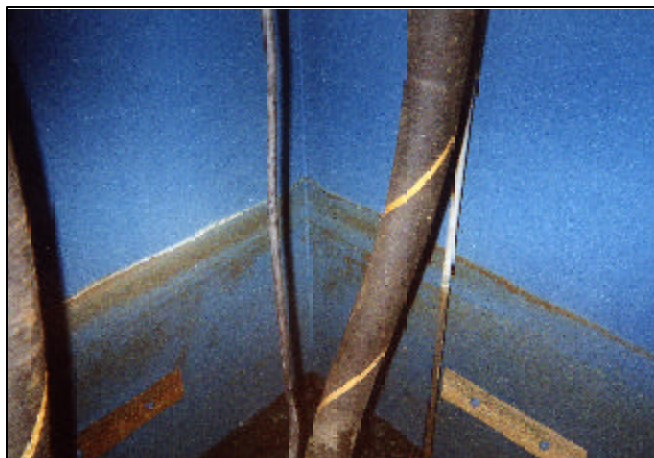
The Inside of the Table Mountain SBR coated with 16 mils (400 microns) of Madison's Corrocote Plus . No evidence of coating breakdown or corrosion whatsoever.
