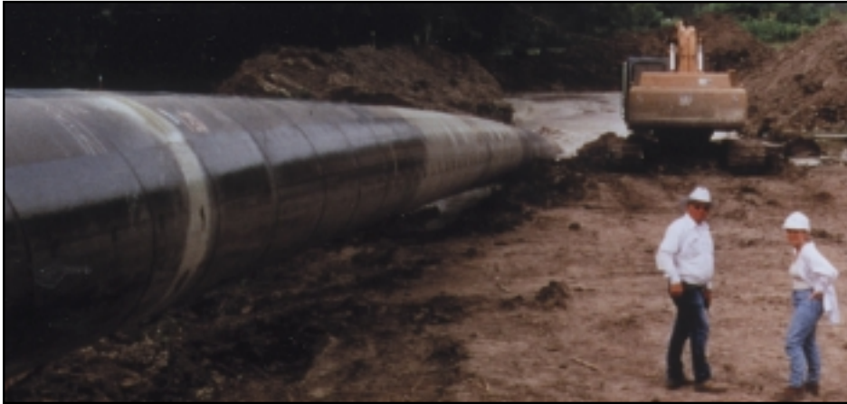
Installation of the world's largest directionally drilled steel pipeline, coated with Madison's Corropipe TX-15 and lined with Corropipe II PW, in Corpus Christi, TX
