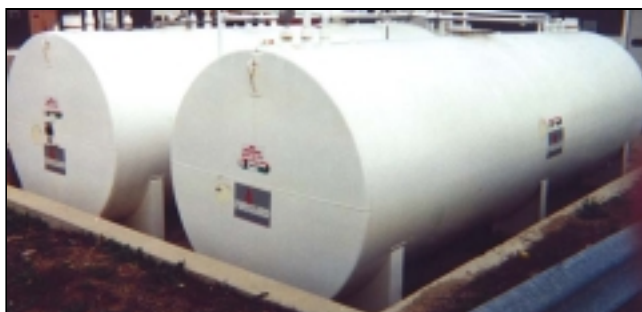
AcrylaThane Coated Fireguard tanks after six years in service storing fuel for the City of Vandalia
