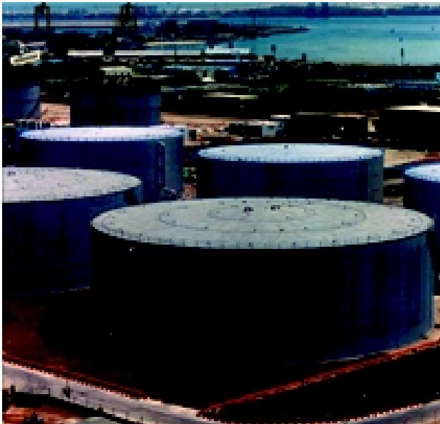
5 million gallon potable water storage tanks lined using Madison's Corrocote II PW in Abu Dhabi, UAE.
