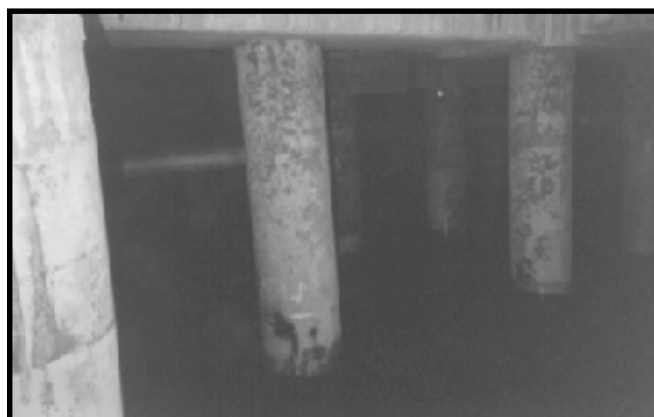
Seriously degraded Fusion Bonded Epoxy coated steel pipe pilings after only six months of service.
