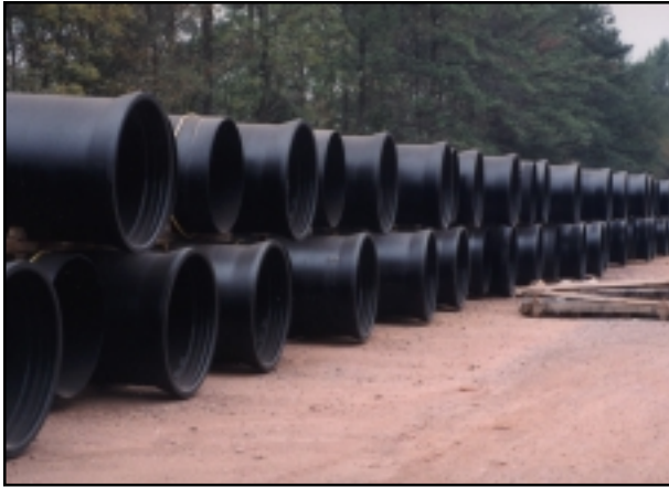
36" Ductile Iron Force Main
