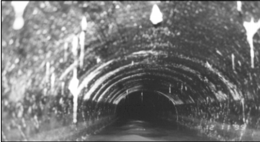
1995 Inspection of sewer line at Rubes Creek Pump Station showed the perfect condition of Madison's coatings.
