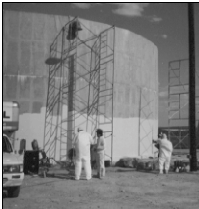
Eagle Pass concrete water tank
