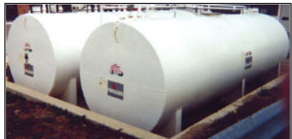
Figure 5 The same two aboveground tanks after 4 years in service
