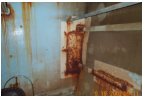
Figure 12. A corroded ballast tank of USS Gunston Hall
