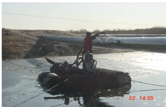
Figure 2. Application of the 100% solids, rigid, aromatic polyurethane coating for river crossing on top of an iced river
