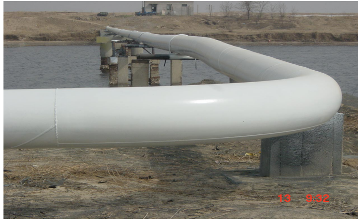
Figure 3. A river-crossing section of the DaGang-CangZhou gas pipeline after being re-coated with a 100% solids, rigid, aromatic polyurethane coating and then top coated with a high solids, UV stable, aliphatic polyurethane coating
