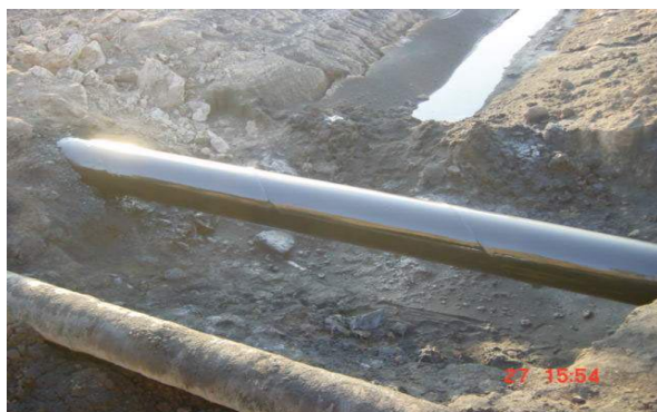
Figure 1. Comparison between a coated and uncoated pipe after 5 minutes of the polyurethane coating application at -15°C (9°F)
