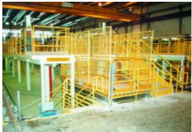
In an aggressive environment such as this commuter rail maintenance facility for the Boston Mass Transit Authority, a duplex system provides superior corrosion protection. All of the exposed steel from the beams to the handrail were hot-dip galvanized and then painted. Proper surface cleaning and profiling ensure the success of this duplex system.
