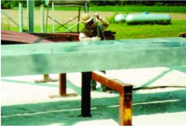
Thorough removal of surface contaminants greatly improves adhesion of the paint to the galvanized surface and is integral to the success of a duplex system.
