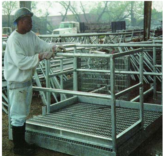
A worker files off a high spot on a piece of handrail. Proper surface preparation is essential for good paint adhesion.
