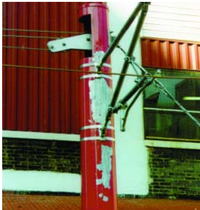
Use of post-treatments, such as water-quenching, can undermine the success of a duplex system by causing adhesion failure, as illustrated by the peeling paint on this pole.
